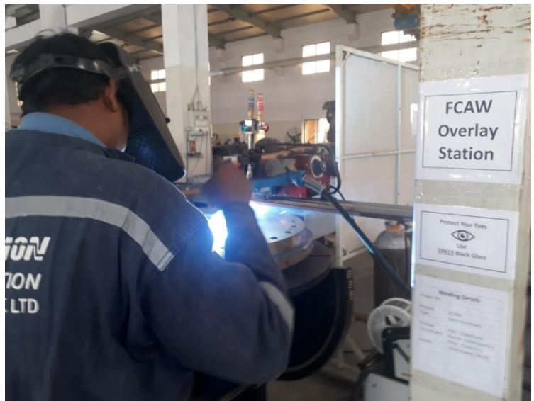
Fully Equipped MIG / FCAW Overlay Station
